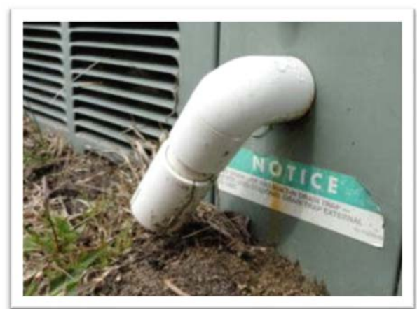
Air Conditioning Condensation
