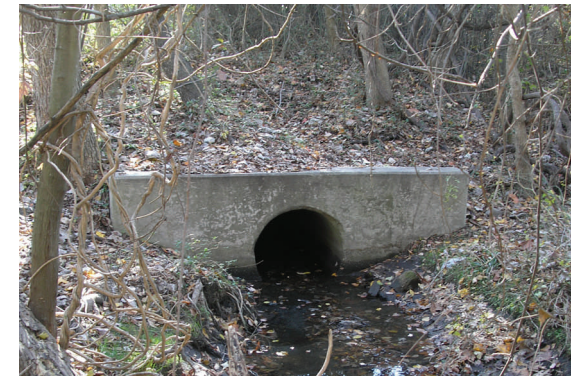
Outfall in a wooded, rear corner of a lot. In such cases, easements are likely recorded on the property and may not be known to the property owner.
